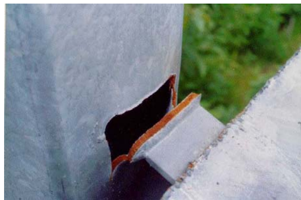
Figure 5.5.3 Base Metal Failure
